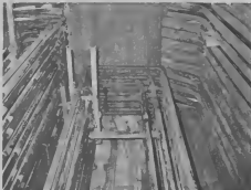
THIS MAZE of piping is connected to the steam drum. E LABIRINTO di tubo aki ta conecta cu drum di stiem.
